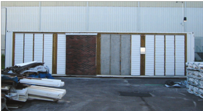
Relocatable Building Enclosure Test Station (RBETS) units were designed and built to test wall assemblies and their component materials in a variety of climates.
