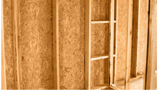
Ladder junctions at interior-exterior wall intersections (Figure 5) produce wall cavities that can be easily insulated to help builders earn the ENERGY STAR® label for new homes.
