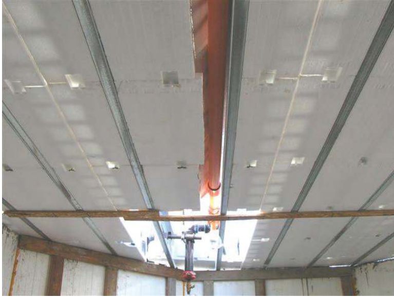
Figure 6.3 – Fire sprinkler system attached to steel joist
