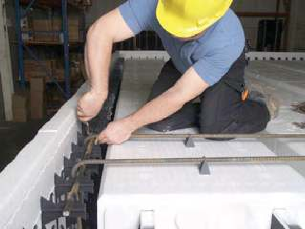
Figure 7.22 - Tying the top slab reinforcement with the horizontal bars on ICF wall
