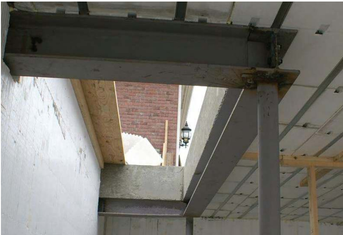
Figure 6.13 – Large sized opening in AmDeck™ supported by steel perimeter beam and column.
