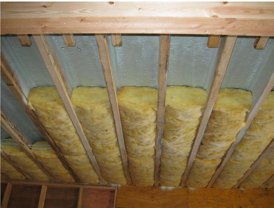
Figure 10. Use a flash and batt approach to insulate and air seal the garage ceiling.
