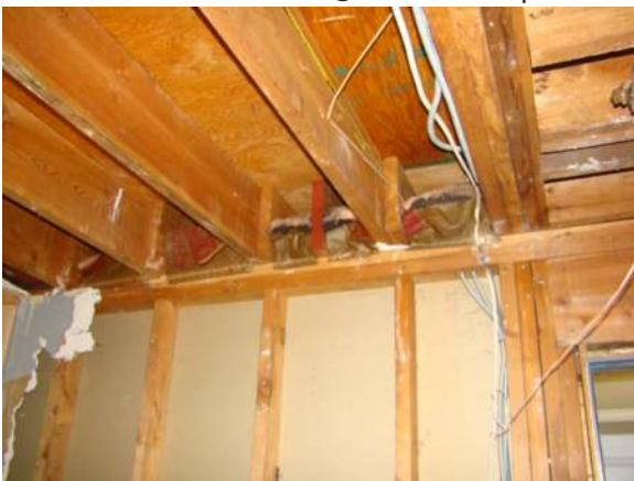
Figure 2. When ceiling joists over a garage run perpendicular to the adjoining wall, the joist bays must be blocked and sealed to prevent garage fumes from entering the living space. (Image courtesy of CARB)
