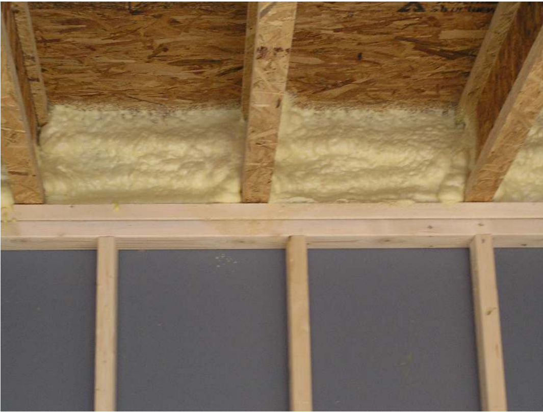
Figure 9. Spray foam insulates the rim joist and air seals the subfloor-rim joist and rim joist-top plate connections.
