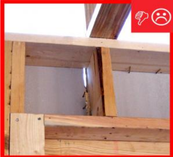
Display Image: TE441_rigidfoam_wrong11_JC2006.jpg Courtesy Of: PNNL
