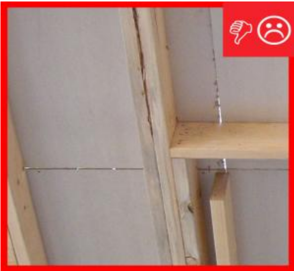
Display Image: TE441_rigidfoam_wrong9_JC2006.jpg Courtesy Of: PNNL
