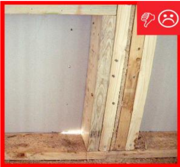
Display Image: TE441_rigidfoam_wrong12_JC2006.jpg Courtesy Of: PNNL
