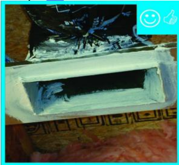
Display Image: HVAC221Flex-R3_BSC06.jpg Courtesy Of: BSC
