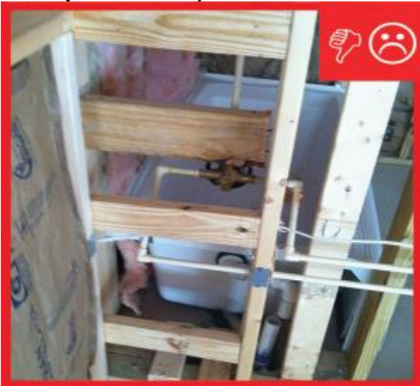
Display Image: JM_behind-tub-missing-air-barrier-3_wrong_TE.jpg Courtesy Of: Jim Mackovyak
