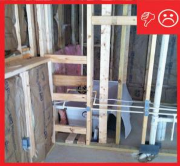
Display Image: JM_behind-tub-missing-air-barrier-1_wrong_TE.jpg Courtesy Of: Jim Mackovyak
