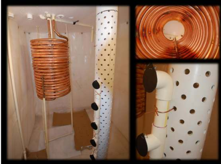
Figure 7: Heat exchangers inside a custom built tank transfer heat to the water in the storage tank. The copper coils transfer heat from the masonry heater, and the white piping transfers heat from the solar thermal panels. The white pipe is perforated to place heated water at a depth in line with the tank's stratification. Photo courtesy of REINA, LLC.
