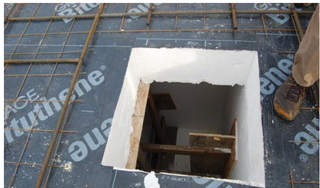
Figure 6: A man-hole looks down into a 1500-gallon tank under construction underneath a house foundation.
