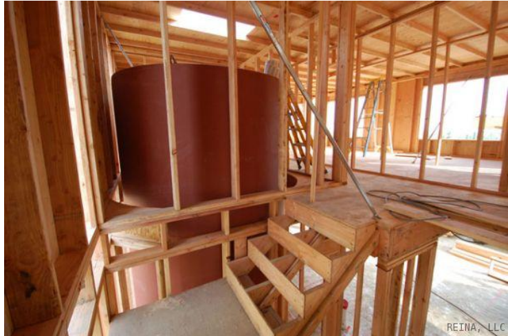
Figure 5: A 5000 gallon tank sits in the middle of a home heated by a solar thermal system. Photo courtesy Reina, LLC.
