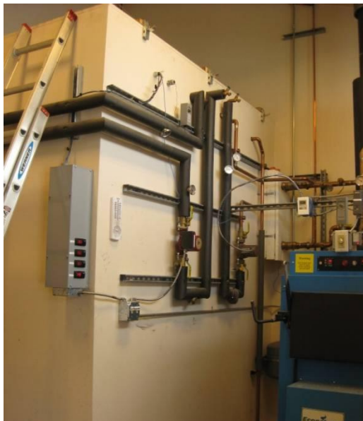
Figure 4: CCHRC's wood-fired boiler sits next to a 1500 gallon storage tank of water.
