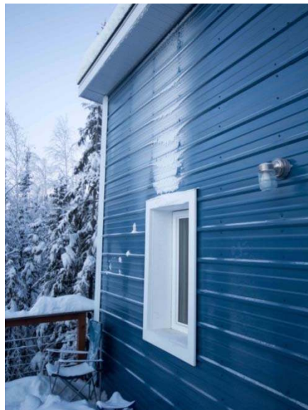
Figure 12. Frost formation above the window was created by the vapor escaping from the open window in the Spruce house.
