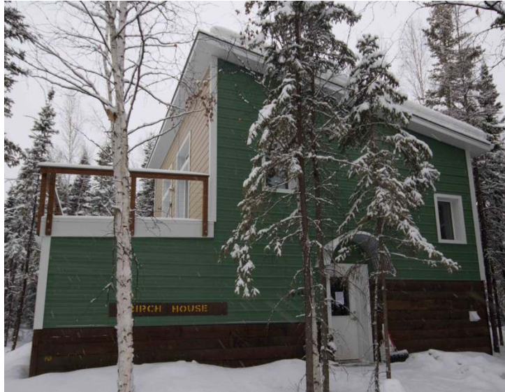
Figure 4. Birch house. This house has 5.5 inches (14 cm) of fiberglass batt in the stud space and 8 inches (20cm) of rigid polystyrene foam on the outside of the sheathing.
