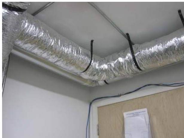
Figure 3: This photo shows an air duct attached to the ceiling. The duct carries heated air above the door of a mechanical room and delivers it to rooms in the house.
