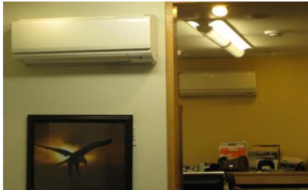
Figure 4: Two indoor units of a mini-split ductless heat pump system appear in two rooms of a building. The indoor units have a fan that blows air over coils containing heated refrigerant and into the room.
