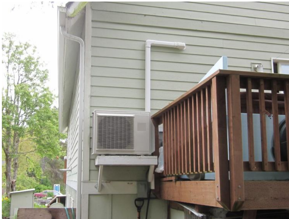
Figure 10: The outdoor unit of a DHP is located next to the porch behind a house. Photo courtesy of Craig Moore.
