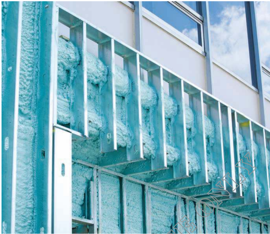
In the photo above, SPF has been applied under a cantilevered wall section.
