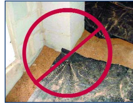
Do not leave any exposed earth in the crawl space! Photo credit: Bill Warren.
