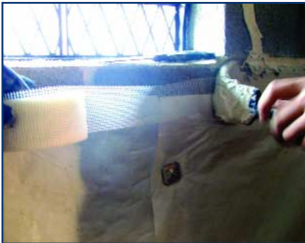
This heavy-duty vapor retarder material is mechanically supported by metal pins with cap washers and sealed to the masonry with fiberglass mesh tape and duct mastic. Photo credit: Indoor Environmental Systems.
