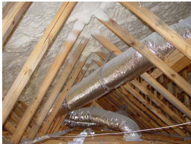
Figure 3 - Unvented attic assembly using SPF insulation (Note: rafters covered to provide layer of continuous insulation) Courtesy of Spray Polyurethane Foam Alliance
