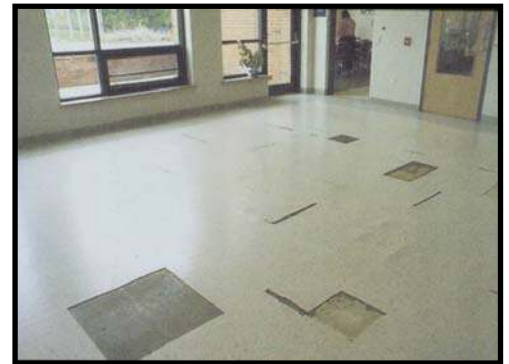
Flooring failures on project above
