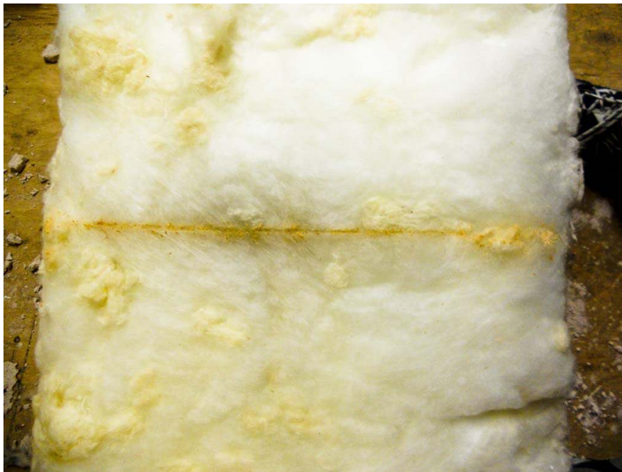
Figure 17. Back of fiberglass from Wall 5. The line in the fiberglass is from the cut that was made in the plywood during construction. The grey discoloration around the line is most likely due to air leakage around the gap in the plywood. Photo courtesy of Randy Nicklas of Icynene.
