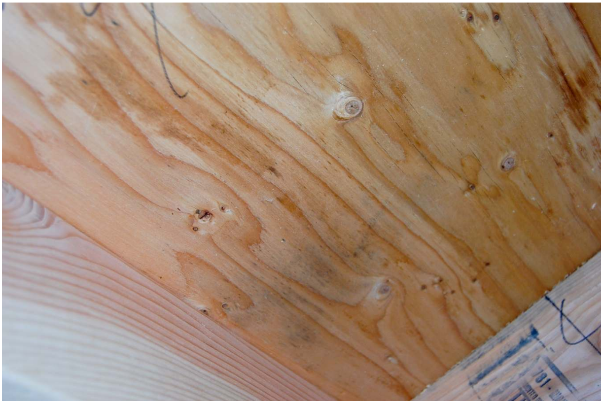
Figure 34. Mold behind the fiberglass of Wall 5. This wall had a several spots of mold on the sheathing that WUFI Bio does not predict.
