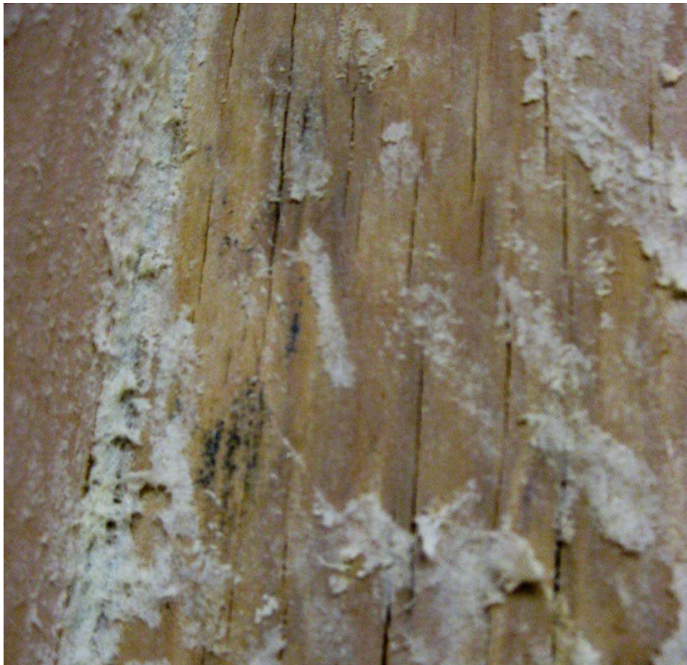
Figure 18. Mold in the upper cavity of Wall 7b. The spot of mold is less than 1 in 2 .
