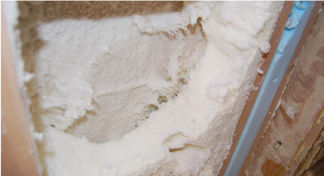
Figure 24. Voids in the ocSPF of Wall 7a. Instead of adhering to the plywood, the ocSPF created an air pocket throughout the lower cavity of Wall 7a. This photo shows the full span of the 15-inch stud cavity.
