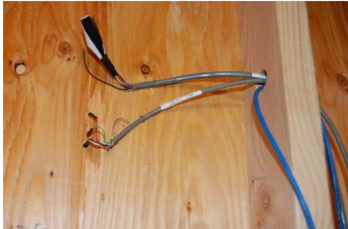
Figure 8. Sensors installed on the plywood sheathing. The relative humidity/temperature sensor is on the top. Below it the moisture content sensor is embedded directly into the plywood.
