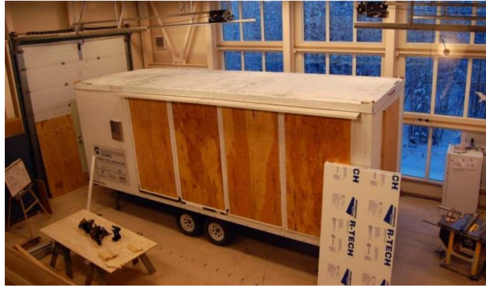
Figure 1. The MTL under construction. The walls for the MTL were constructed inside the building and then the trailer was moved outside to a clearing to the south of the building.
