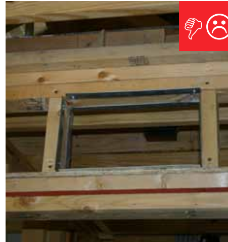
B. Transfer grill not sealed.
