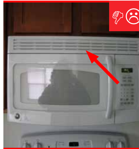
C. Recirculating fan installed that does not exhaust to outside.
