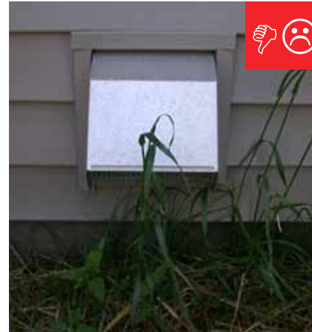
C. Ventilation inlet is too close to the ground and is being blocked by the grass.
