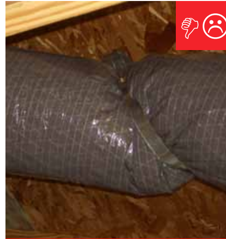
C. Metal strap is too small and is compressing duct.
