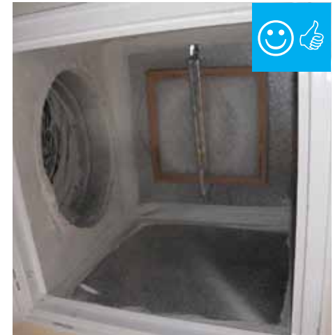
There is a filter installed to filter outdoor air.
