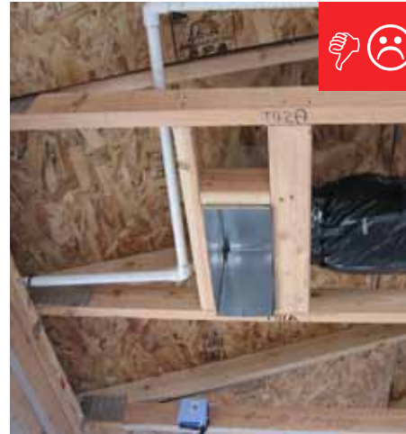
B. Insulation does not cover boot and is not sealed.
