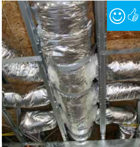
Trunk to duct connections are properly insulated and have been sealed with mastic.
