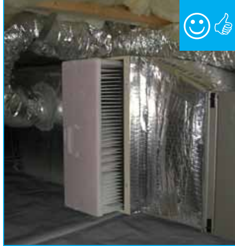
The installed filter is at least a MERV 6 filter.
