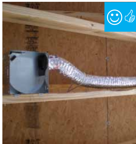
Fan housing was oriented in the correct direction to allow proper exhaust duct installation.
