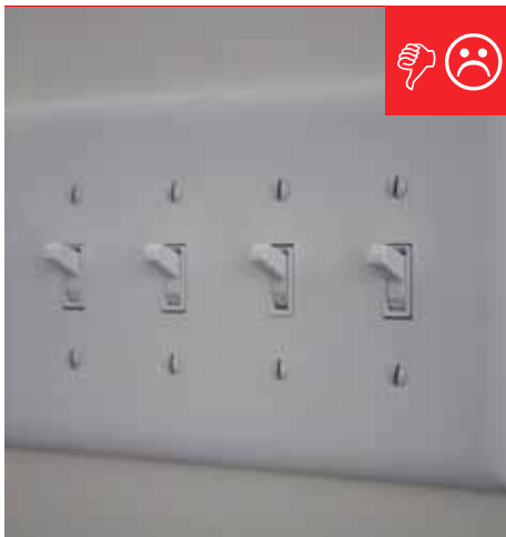
B. Ventilation control is not obvious.
