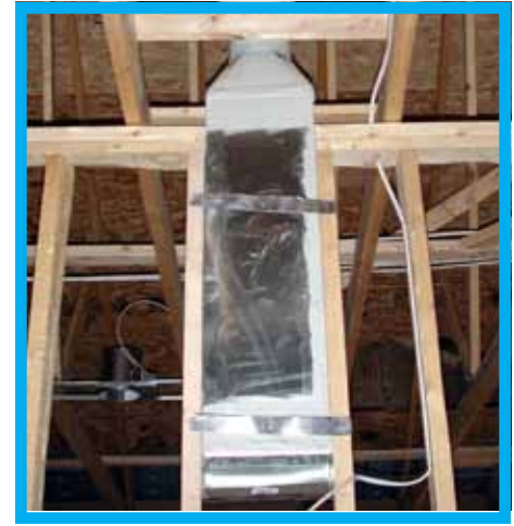
Kitchen exhaust properly installed and sealed with mastic.
