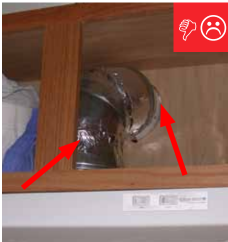
D. Exhaust duct work and penetration to the exterior have not been sealed.
