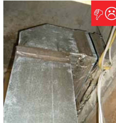
A. Duct work is uninsulated and not sealed at seams.
