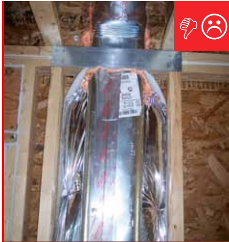
A. Inadequate amount of insulation installed with compression, misalignment, and voids.
