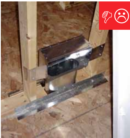
C. No insulation installed in cavity and not air sealed.
