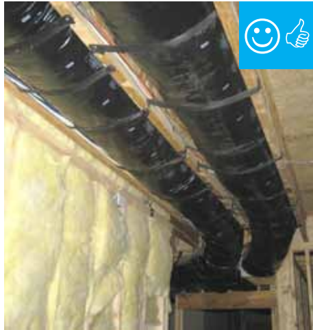
Ducts well supported.
