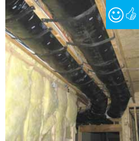
Ducts are properly insulated and supported without compressing the insulation.
