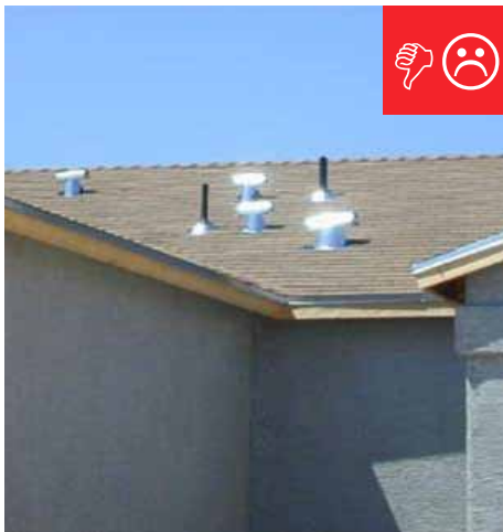
C. Ventilation inlet is too close to exhaust outlets and does not extend at least 2 ft. above the roof deck.
