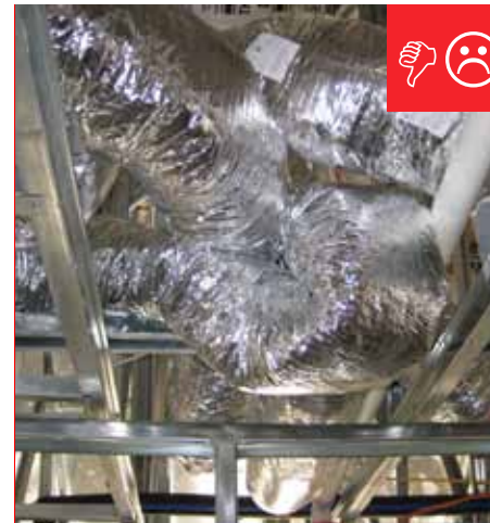
B. Ducts crammed into cavity, kinked and sharply bent.
