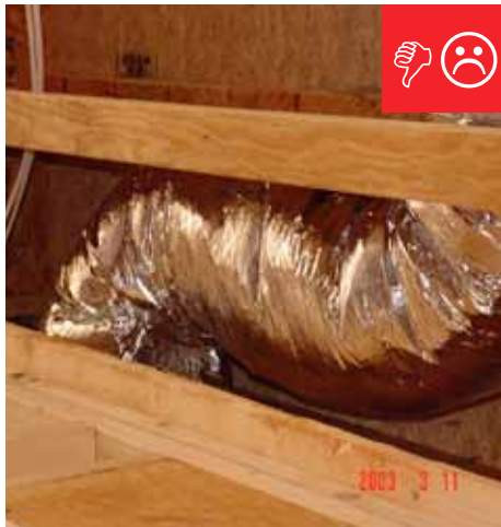
A. Duct is kinked in cavity.
