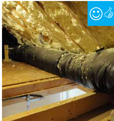
Duct is run straight and supported properly.
