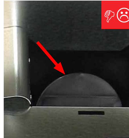
B. Back-draft damper still has a piece of tape that prevented it from rattling during shipping.
