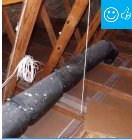
Duct is located in unconditioned space and is properly insulated.
