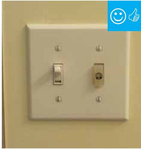
Manufacturer labeled ventilation switch.
