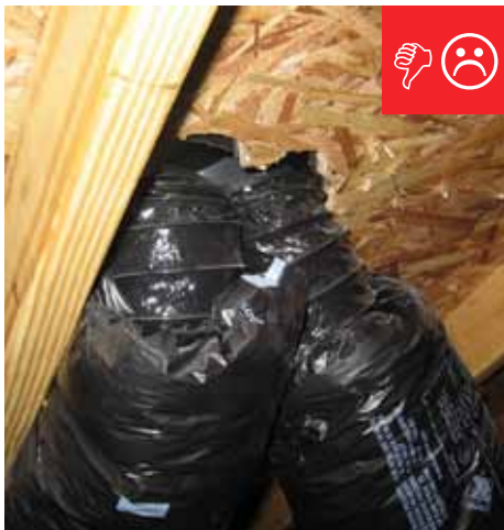
C. Fans from separate dwellings exhausted together without back-draft dampers and not sealed.
