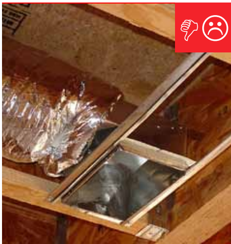
C. Insulation does not cover boot and is not sealed.
