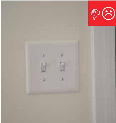
A. Ventilation control is not obvious.
