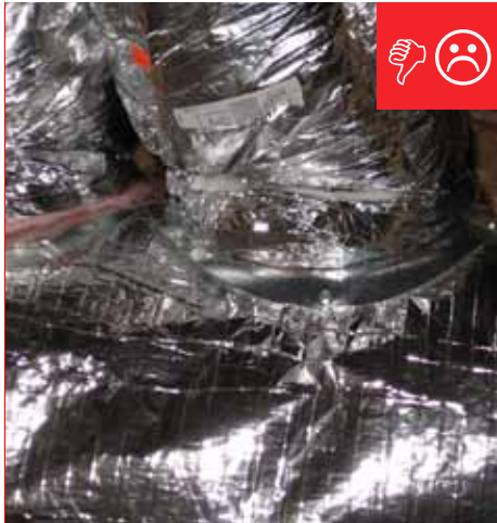
A. Trunk to duct connections are only mechanically fastened and not sealed.
