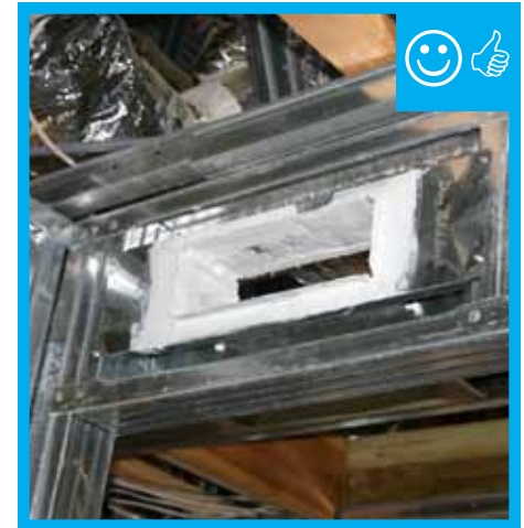
Transfer grill sealed with mastic.
