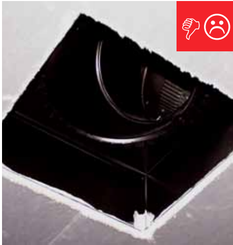
A. Fan shares exhaust and does not have a back-draft damper installed.
