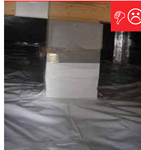
C. The polyethylene sheeting is not staked or attached to furring strips for mechanical support.
