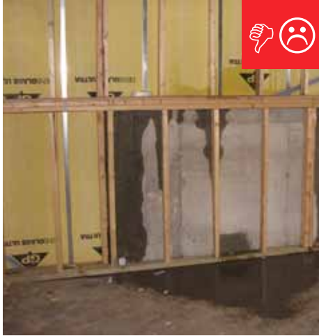
A. Untreated lumber has been used on a below-grade wall against masonry.
