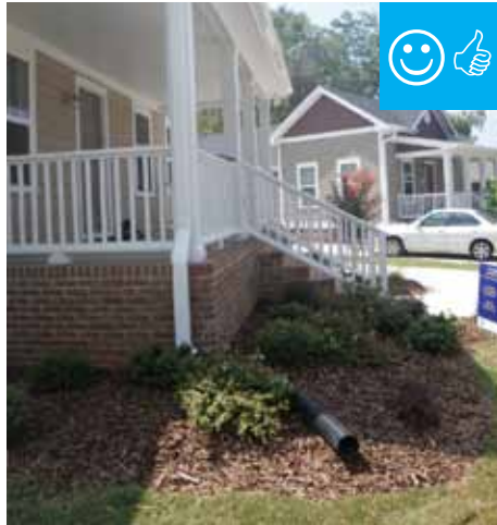
The downspout pipes far enough away from the foundation to prevent moisture problems.
