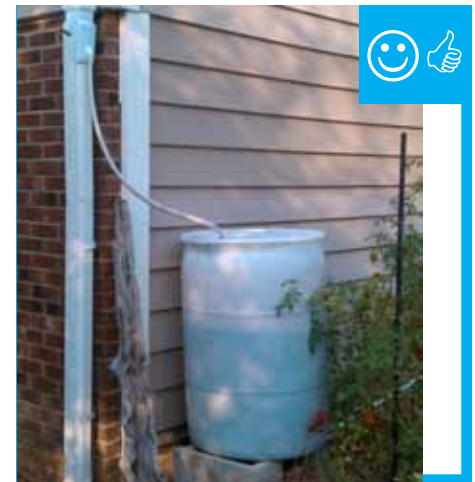
Rain barrel installed with an overflow spout terminating at least 5 feet from foundation.
