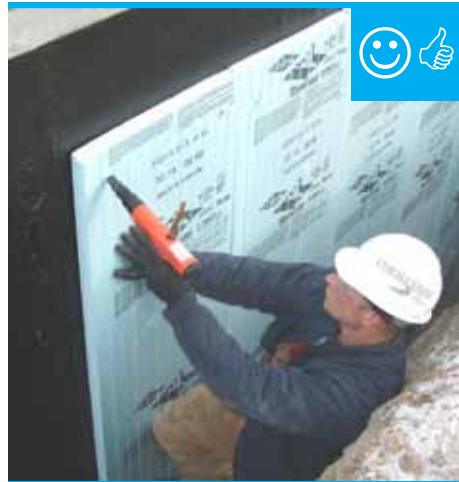
Below-grade concrete has been properly sealed against moisture and is now having insulation installed.
