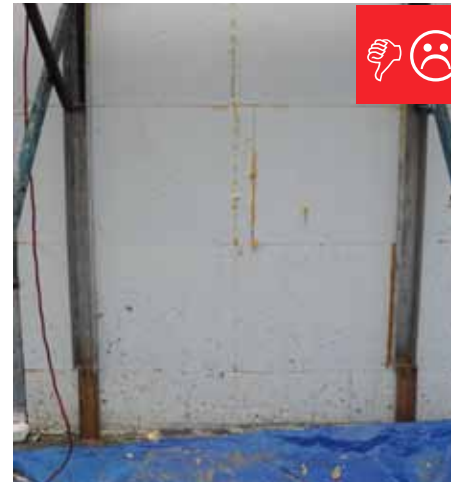
D. The insulated concrete forms at the foundation do not have a damp-proof coating.
