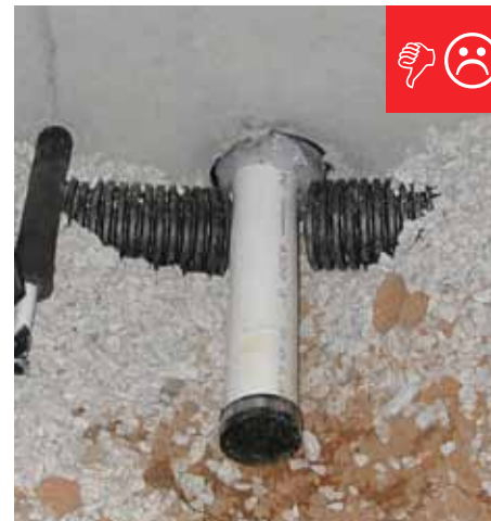
D/H. Drain pipe has been cut and foundation penetration has not been properly sealed.
