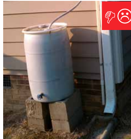
D. Rain barrel installed without an overflow spout that terminates away from foundation.
