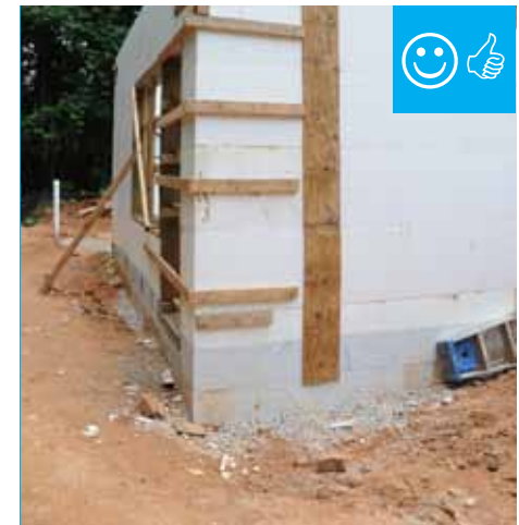
The insulated concrete forms that are below grade have a damp-proof coating to prevent moisture seeping into the foundation.
