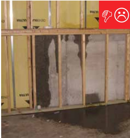
A. The below-grade concrete does not have the correct mixture to be impermeable to moisture.
