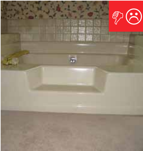
A. There is carpet installed too close to the plumbing fixtures in the bathroom.
