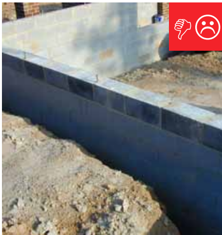
C. The below-grade concrete walls do not have any damp-proof coating.
