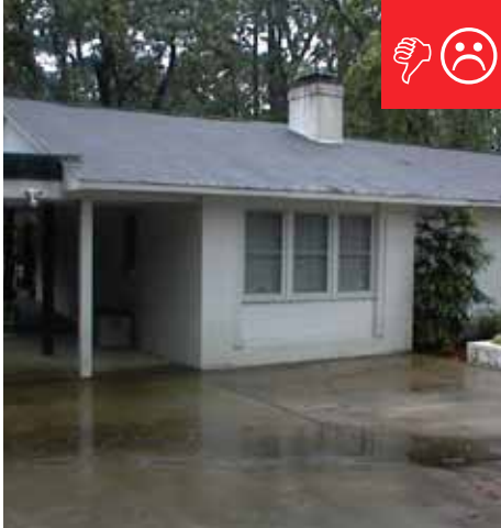
A/B. Driveway is not sloped away from the house.
