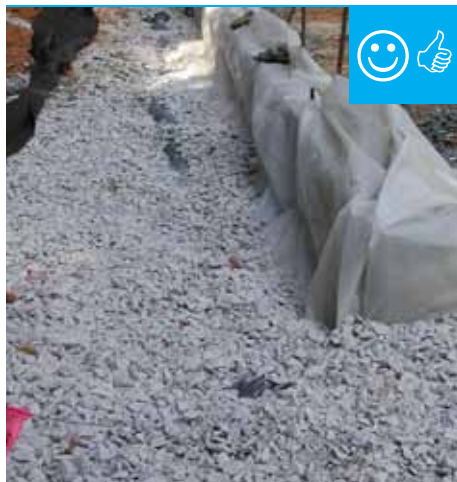
House without gutters has waterproof liner, drain tile and gravel bed extending more than 5 feet from foundation.
