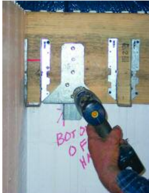
Figure 8.52 – Installing the ICFLC-W around the ledger board and drilling self tapping screws in the designated holes through to the ICFLC piece
