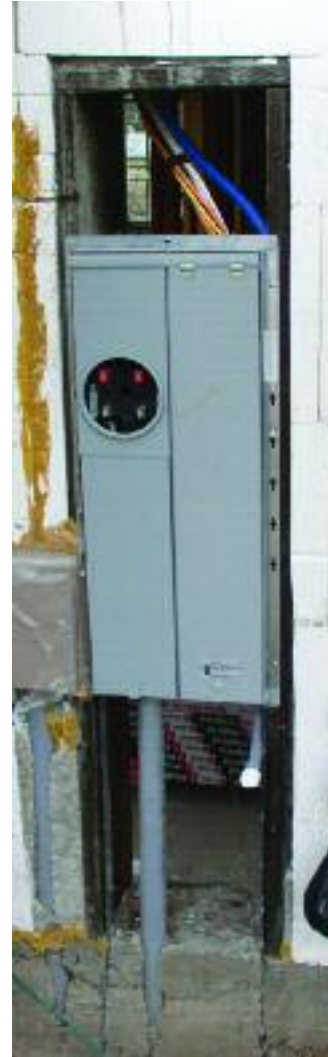
Figure E1.1 – Main electrical panel installed flush with exterior wall
