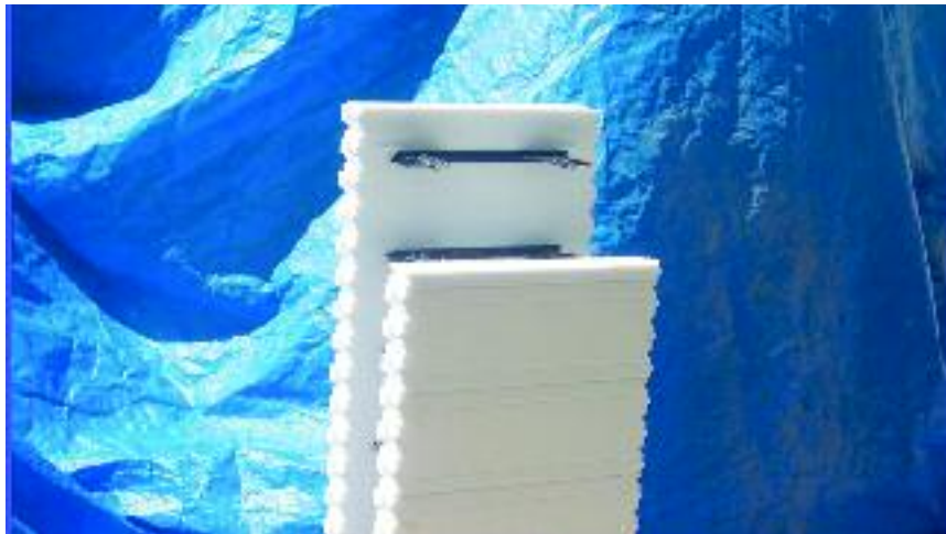
Figure 9.4 – Cutting foam from the end of the straight block on one EPS panel
