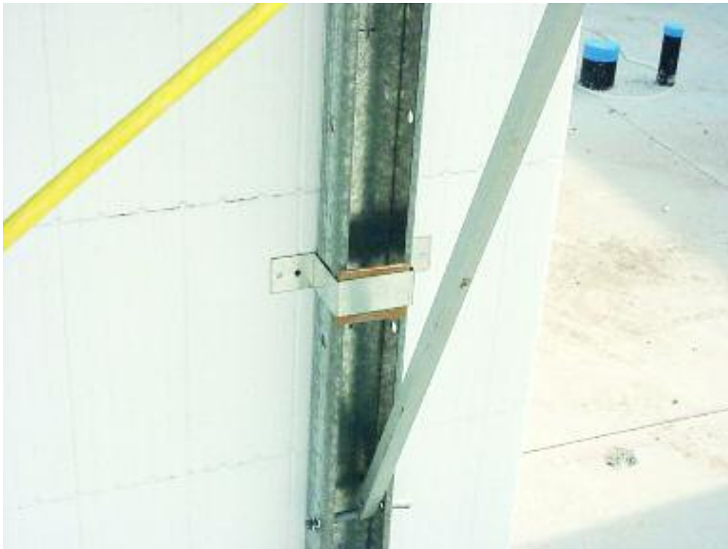
Figure 8.31 – A hat bracket wrapped around a vertical strong-back and screwed to webs on both sides
