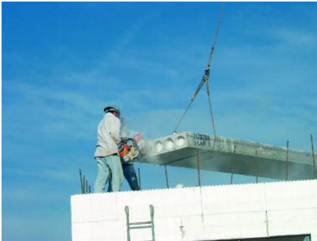
Figure 9.30 – Maneuvering a pre-cast hollow core slab for placement on an ICF wall
