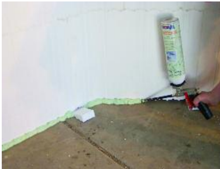
Figure 8.21 – Foaming under a large, low spot area
