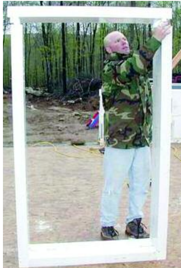
Figure 5.15 – Installing the header. (Hole for pouring concrete not shown.) Image courtesy of V-Buck
