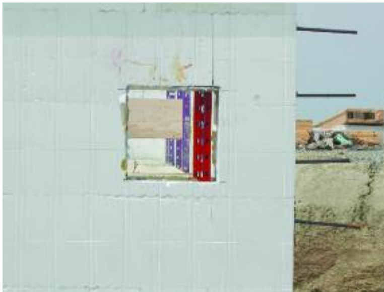
Figure 8.54 – Cut out opening from the inside and outside EPS panels on one side
