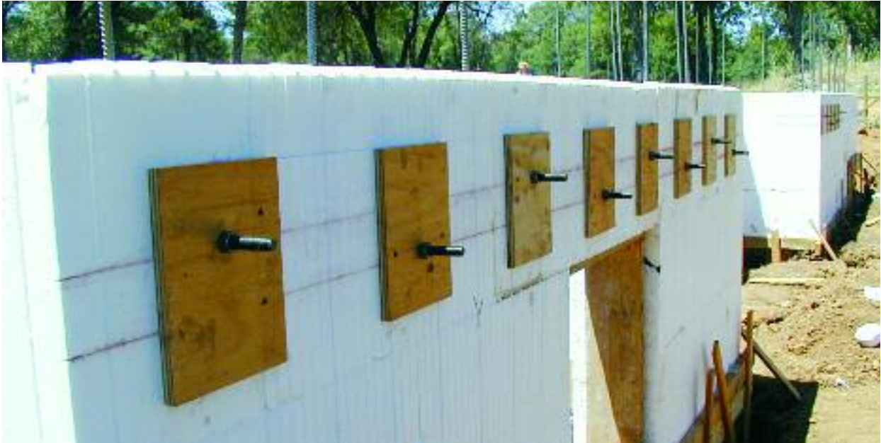
Figure 8.45 – Installing the OSB with anchor bolts onto the EPS openings and securing with sheet rock screws
