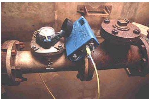
Meter-Master flow recorder installed on a magnetic drive water meter. (Photo courtesy of the F. S. Brainard Company)
