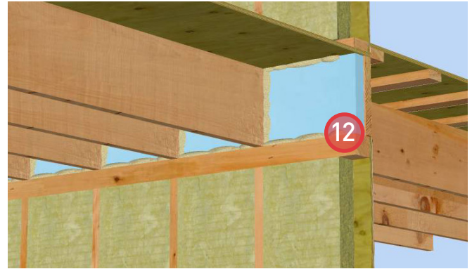
12. Install 2 lb. closed-cell spray or sealant around the perimeter of the rigid insulation to ensure air tightness and thermal barrier continuity.
