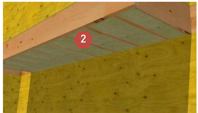
2. Install ROXUL® COMFORTBATT® in the cantilevered floor joist cavities. Ensure insulation extends through to the interior plane of the wall assembly to maintain thermal continuity.
