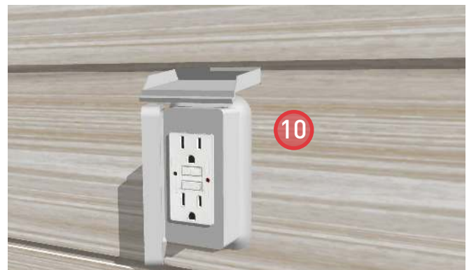
10. Install sealant around the perimeter of the electrical box (top and sides).
