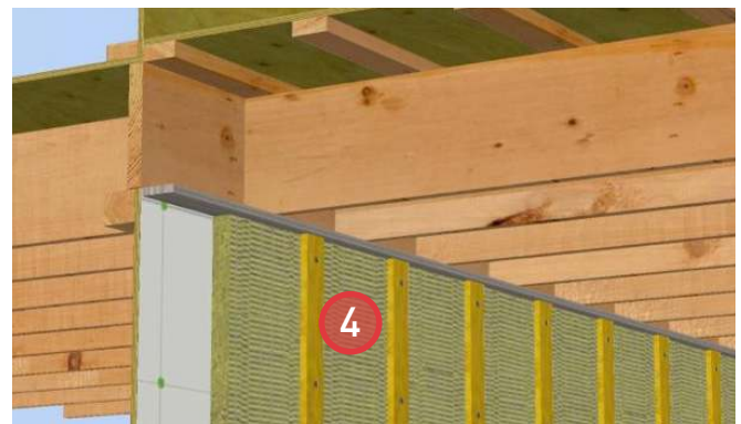
4. Install ROXUL® COMFORTBOARD™ IS and strapping with bugscreens, leaving a \frac{3}{4} " gap between the insulation and the top of the wall. Suggest using a 1x4 temporary spacer board to space the insulation.
