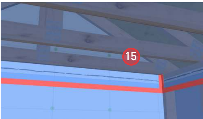
15. Install poly to the underside of the roof framing and fasten with staples at the sealant bead to complete the air seal. Seal the leading edge with sheathing tape.
