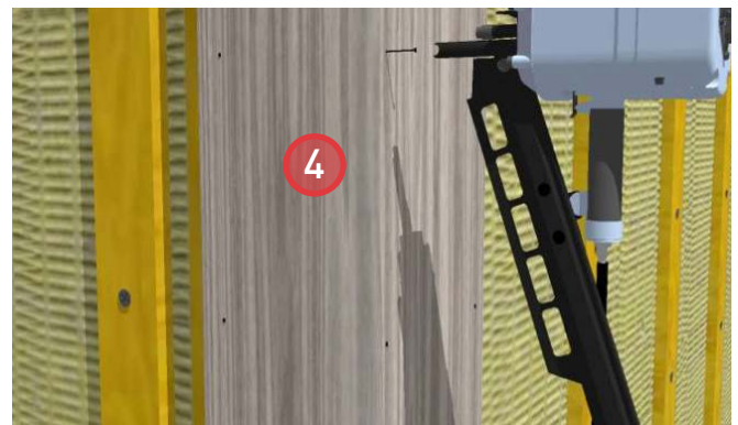
4. The corner trim boards must be nailed together as well as to the strapping to form the corner.
