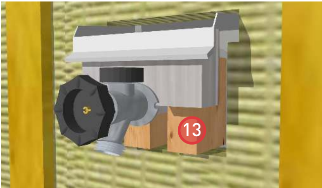
13. Install the top piece of the wood face plate and secure in place.
