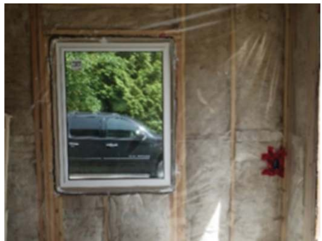
Typical polyethylene plastic sheet (Class I vapour retarder) installed on the interior of a 2x6 insulated wall in Canada
