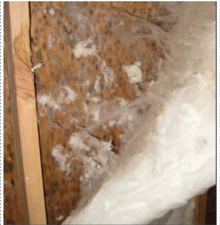
Figure 2. Mold on the sheathing behind the fiberglass on a wall with thin exterior insulation.
