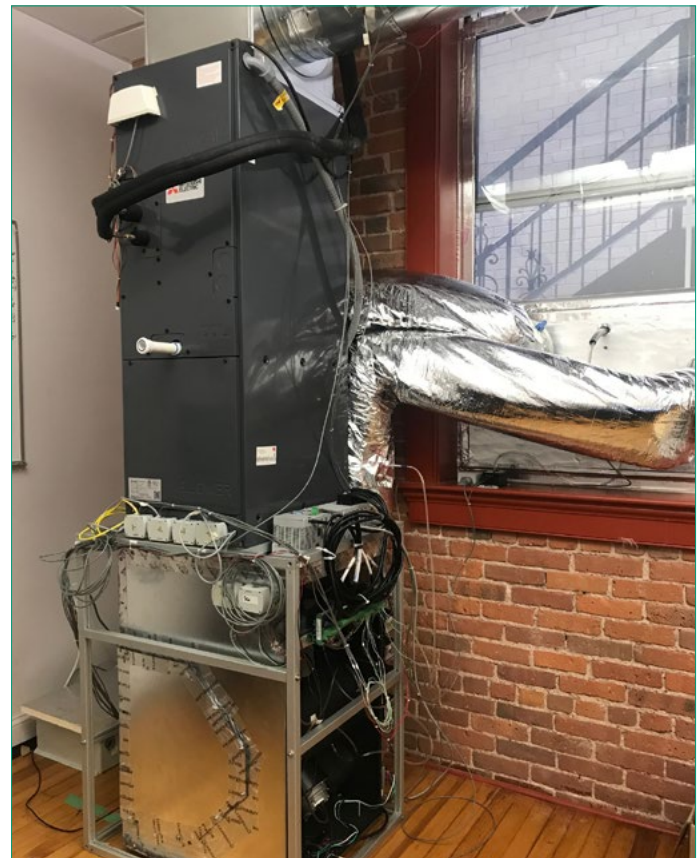
Figure 7. Integrated energy recovery ventilator unit undergoing monitored testing in the Steven Winter Associates, Inc. office. Image courtesy Steven Winter Associates, Inc.
