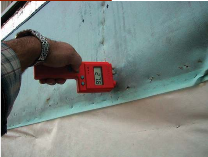
Low vapor permeable housewrap with high moisture reading on OSB under housewrap
