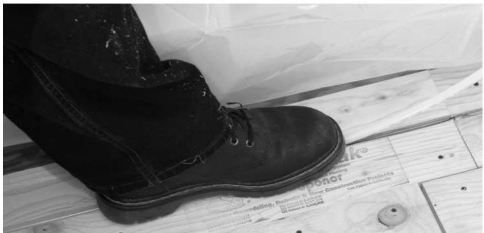
Figure 29: Use hard-soled boots or shoes to walk the tubing into the panel groove.
