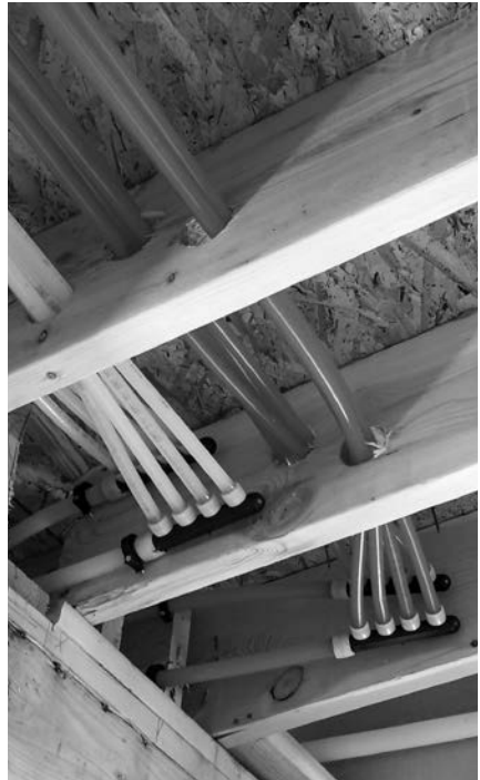
Figure 5-7: Bundled Uponor AquaPEX pipe
