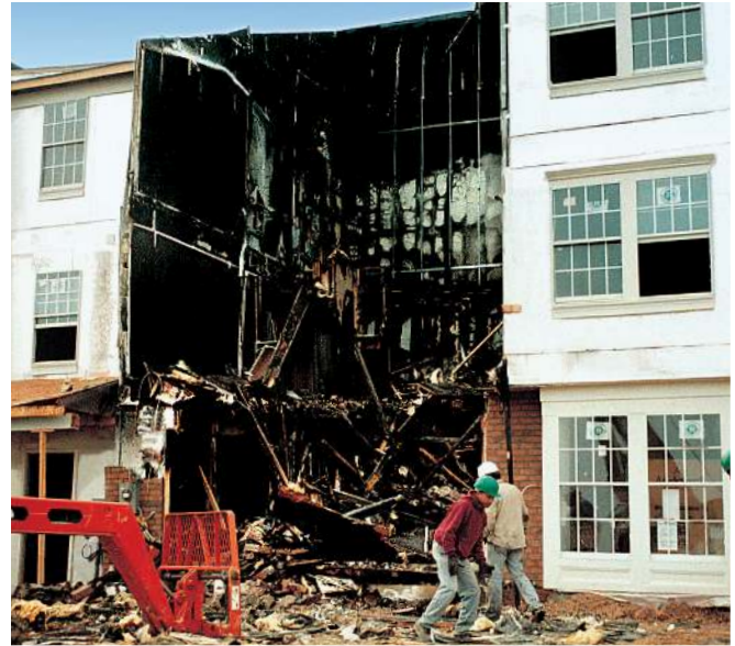
The fire-protection of gypsum-based Area Separation Fire Walls is demonstrated in dramatic fashion by the results of this actual townhouse fire in which the two-hour fire-rated assembly performed as expected in protecting adjacent properties. Break-away feature allowed collapse of fire-side structural framing without pulling down the entire wall.
