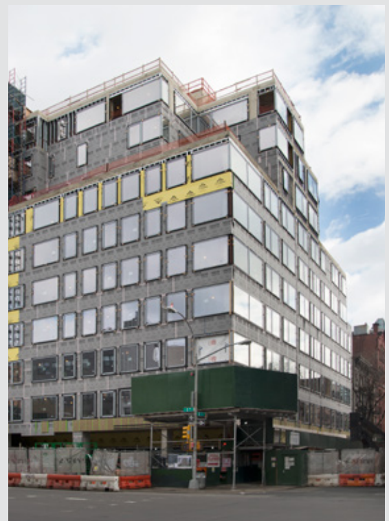
Airtightness is critical for building performance and occupant comfort, and an important component when considering energy efficiency
