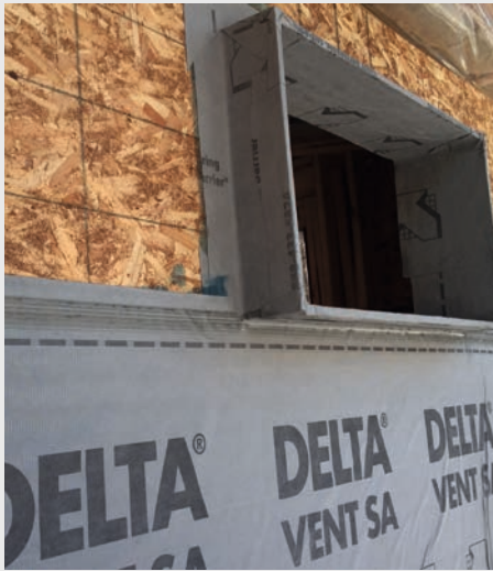
Blower tests confirmed that there were no leaks.
